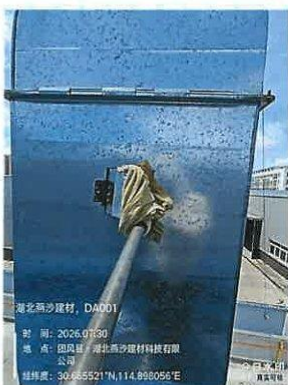
①混料废气排气筒DA001
