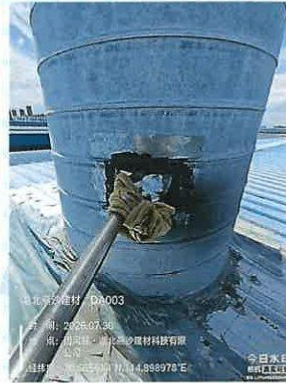
◎3切边、刮平、抛光废气排气筒DA003
